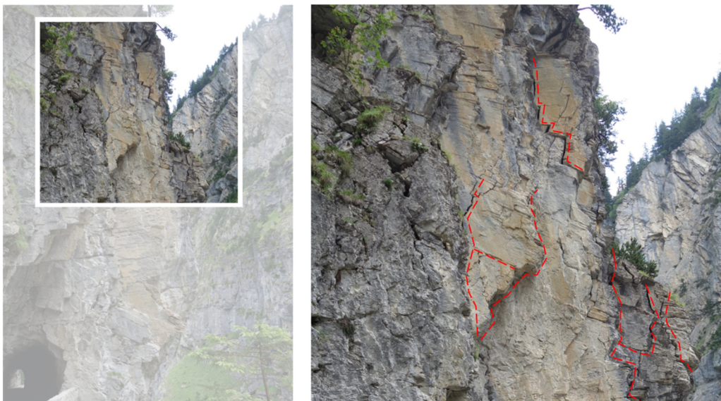
Illustration 18: Analysis of the rock surfaces. At the right side of the photo there is an enlarged section of a rock face at the entrance of a tunnel. The orientation of the fissures (red lines) define the diameters of blocks and stones prone to rockfall. Source: SRC.
