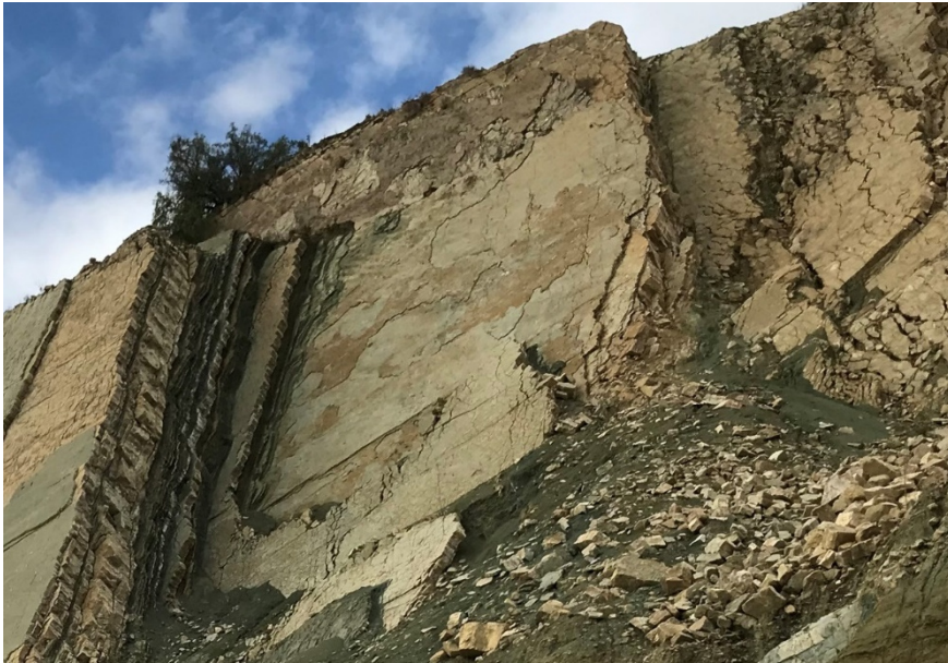
Illustration 17: Analysis of the rocky surfaces. The rock face has a very steep stratification parallel to the slope (left side). The right portion of the photo shows the fractures that cross the strata and, therefore, define the size of the rockfall components.
