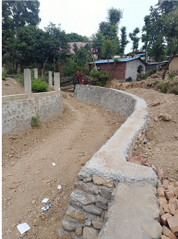
Illustration 7: Riverbank protection wall to protect buildings from floods. Birendranagar, Nepal.
